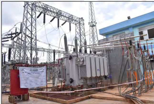
The Mohanpur Sub-station in Tripura...
