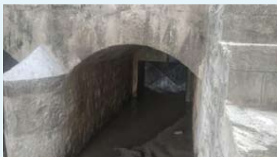
(a) Tunnel type Outlet at Chaparwada Dam (Available head 4 m)
