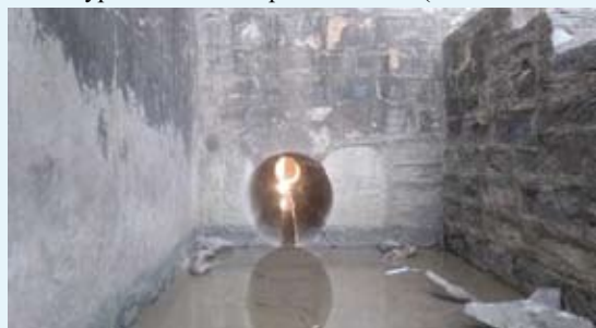
(b) Pipe type outlet at Tordi Sagar Dam (Available head 10 m)
