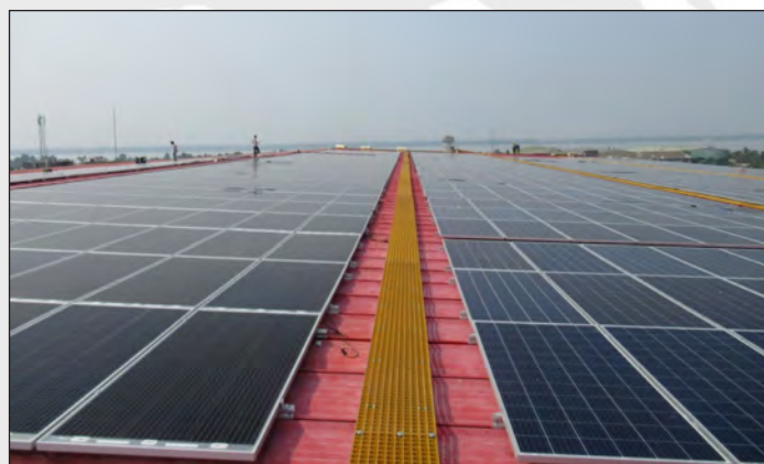
Solar plant in Vikram Solar's Falta plant...
