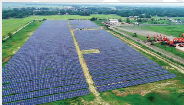
The onsite solar power unit at Tata Hitachi's plant...
