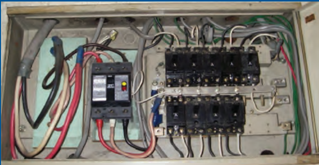
Power distribution panel with loosened screws (digital camera)
