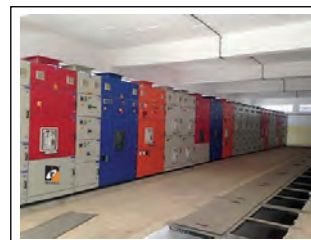
Electrical Control Panel
