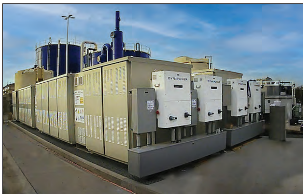
Redflow Energy Pods deployed at Anaergia's Rialto Bioenergy Facility in California...
