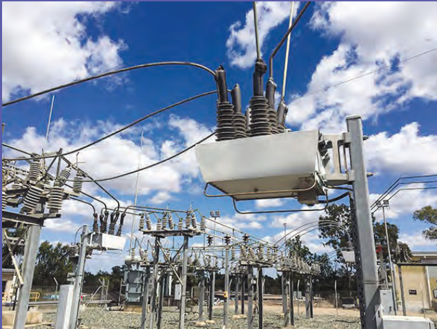
NOJA Power OSM Recloser in a Mining Substation... © NOJA Power 2021
