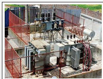
7500 kVA Built in AVR
