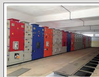
Electrical Control Panel
