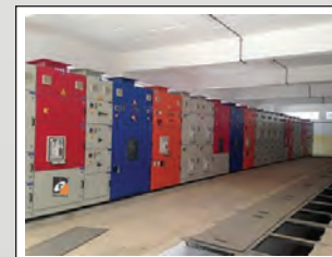
Electrical Control Panel
