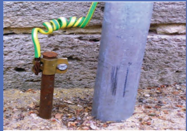
An ideal earthing system The size of the pipe used for earth is of 3.8cm diameter and 2.5m in length. More than 2 meters of the rod is buried in the 'earth pit'. Pit is filled with mixture of powdered coal, salt and sand. Care should be taken to keep the soil of the pit wet.
