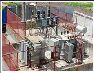
7500 kVA Built in AVR
