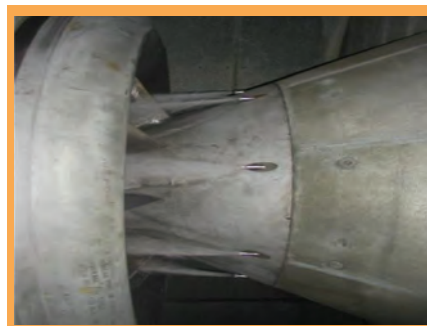
Figure 4: Compressor washing nozzles in operation
