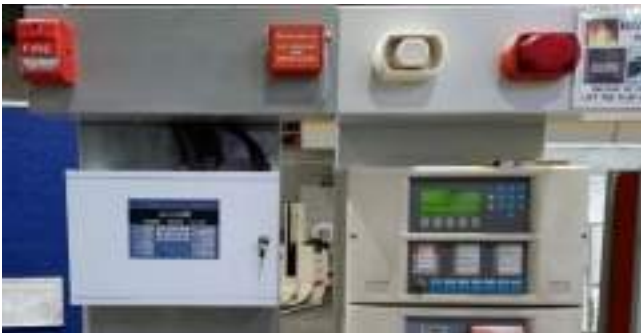
Fig. Automatic CO 2 fire suppression system on all rotogravure printing machines. In case of any incident involving CO 2 release, the machine power automatically shuts down and also activates Fire Alarm Control Panel (FACP) system of the factory.
