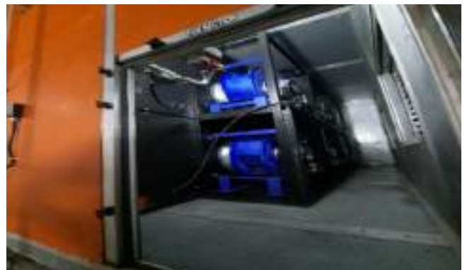
Fig. Unit has changed axial fans for all Air Handling Units (AHUs) to BLDC fans leading to reduction in the energy consumption in AHUs by about 43%
