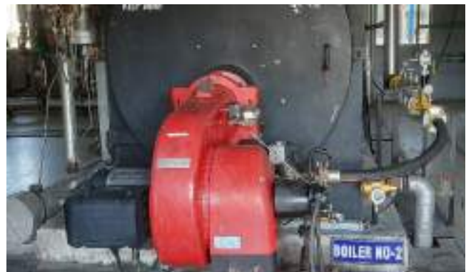
Fig. Unit has undergone the fuel change for thermic heaters and boilers from High Speed Diesel (HSD) to a much cleaner fuel-'propane' to reduce GHG emissions
