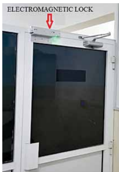
Fig. 5: Electromagnetic lock installation on a glass door
