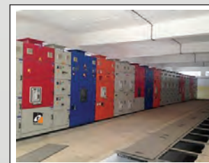
Electrical Control Panel
