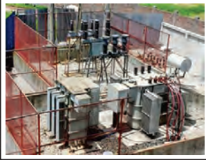
7500 kVA Built in AVR
