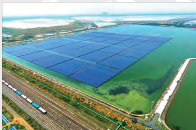
A view of the Ramagundam Floating Solar Project...
