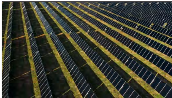
Armadillo Solar Center in Navarro County, Texas...
