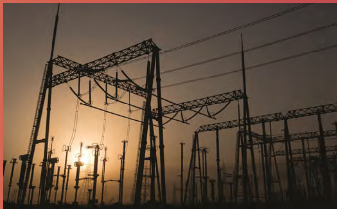
Jharsuguda thermal power plant's switch yard...
